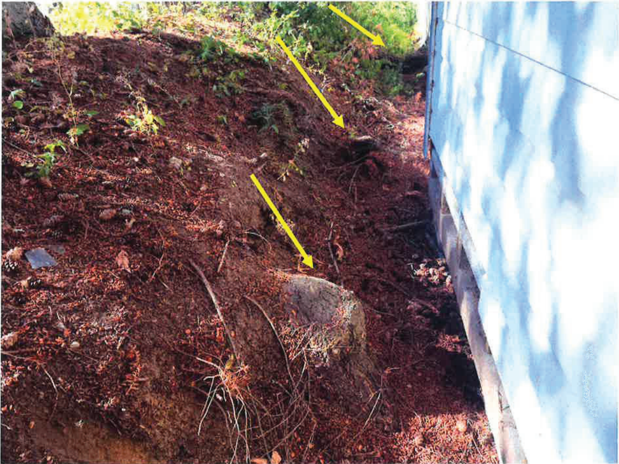
Photo #6 – Exposed Surface Roots – Edge of Annex Building
