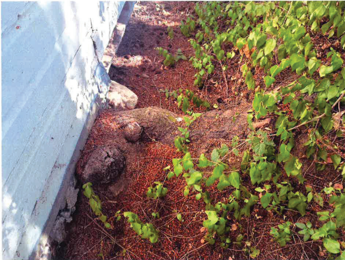
Photo #5 – Exposed Surface Root – Edge of Annex Building
