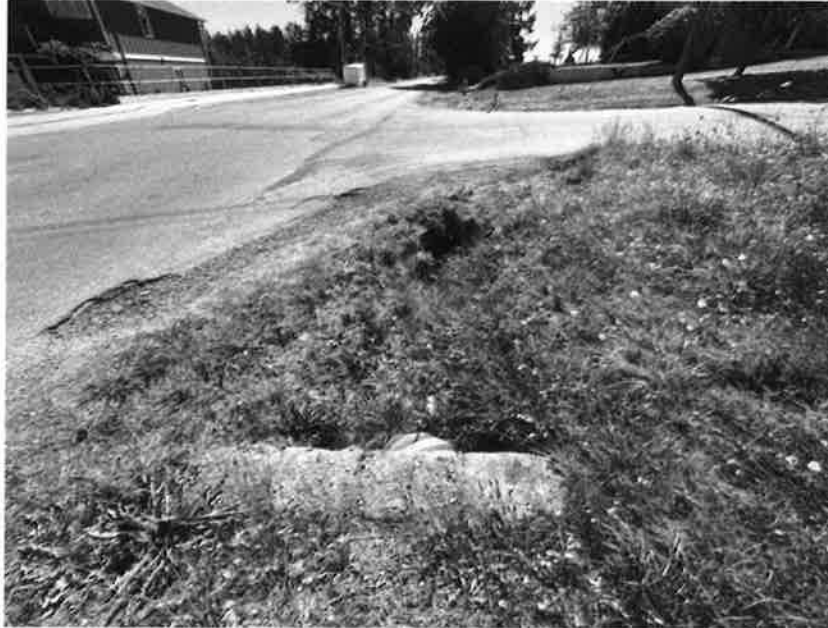
Photo 1. Roadside ditch and culvert at the eastern property extent, looking south (downstream). September 7, 2022.
