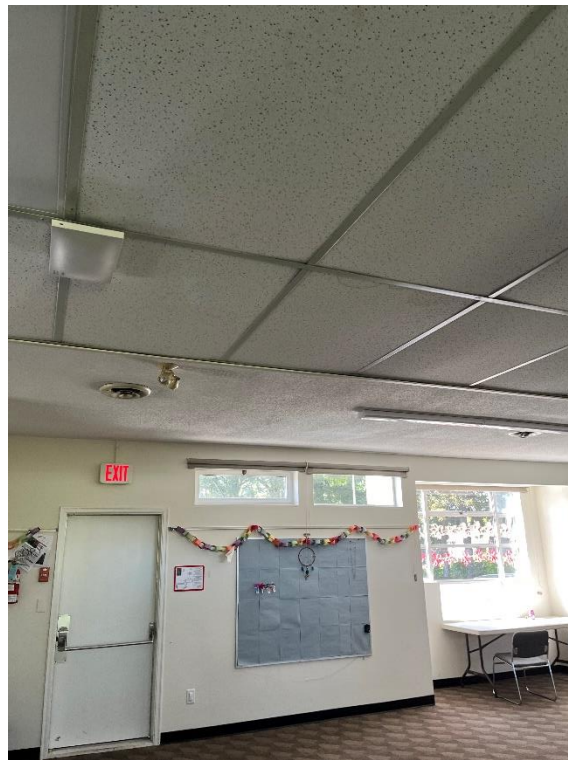
Figure 2: North Activity Room (Showing Ceiling Terminal Units)
