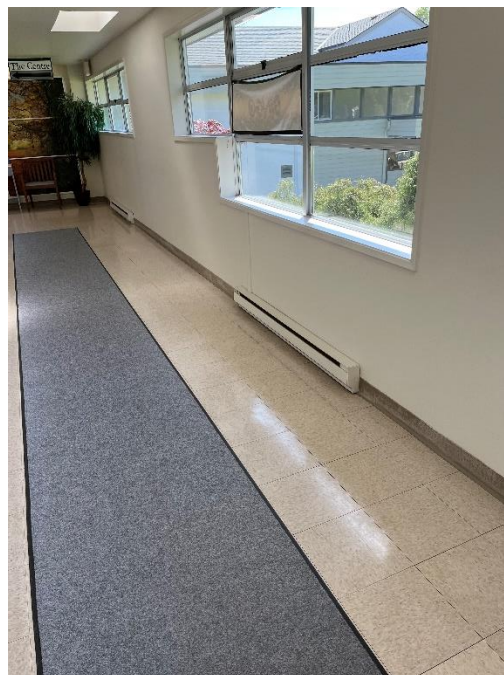
Figure 3: Typical Baseboard Heaters
