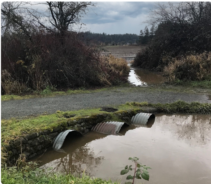
Above: Flooding in Maber Flats/TIKEL
